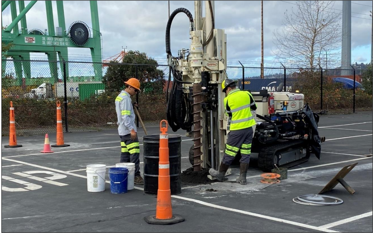
Figure 7. Drilling MW-14 with 6-inch auger and shoveling spoils for inspection. View northwest.
