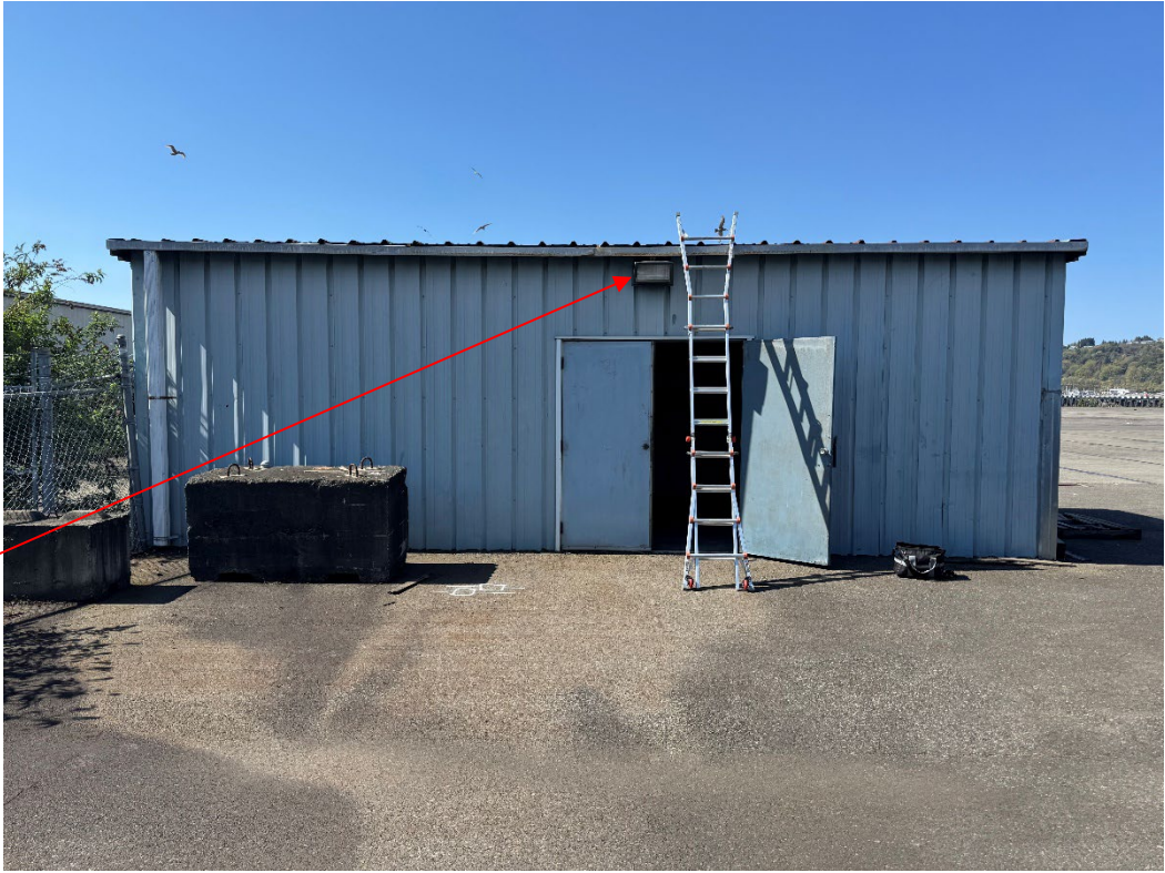
Photo 1 - Shed (12'W x 30'L x 10'H) to be demolished on EBC Tenant Property.
