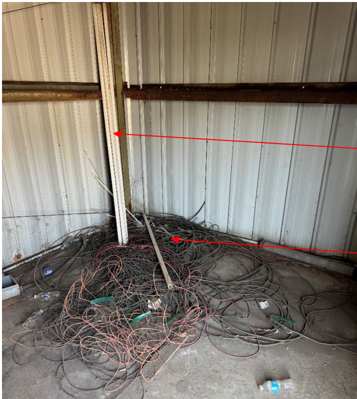
Photo 5 – Pile of non-ACM wire, along with 8' mercury containing fluorescent light tubes. 1 broken tube in corner over lights.
