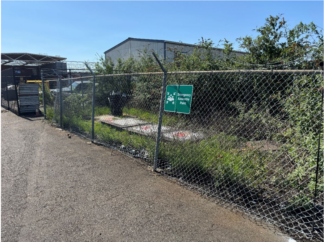
Photo 2 - Fenced area SW of Shed with former transformers, non-ACM power leads connected to vaults under Shed, and other exterior utility vaults. No ACM found in this area.
