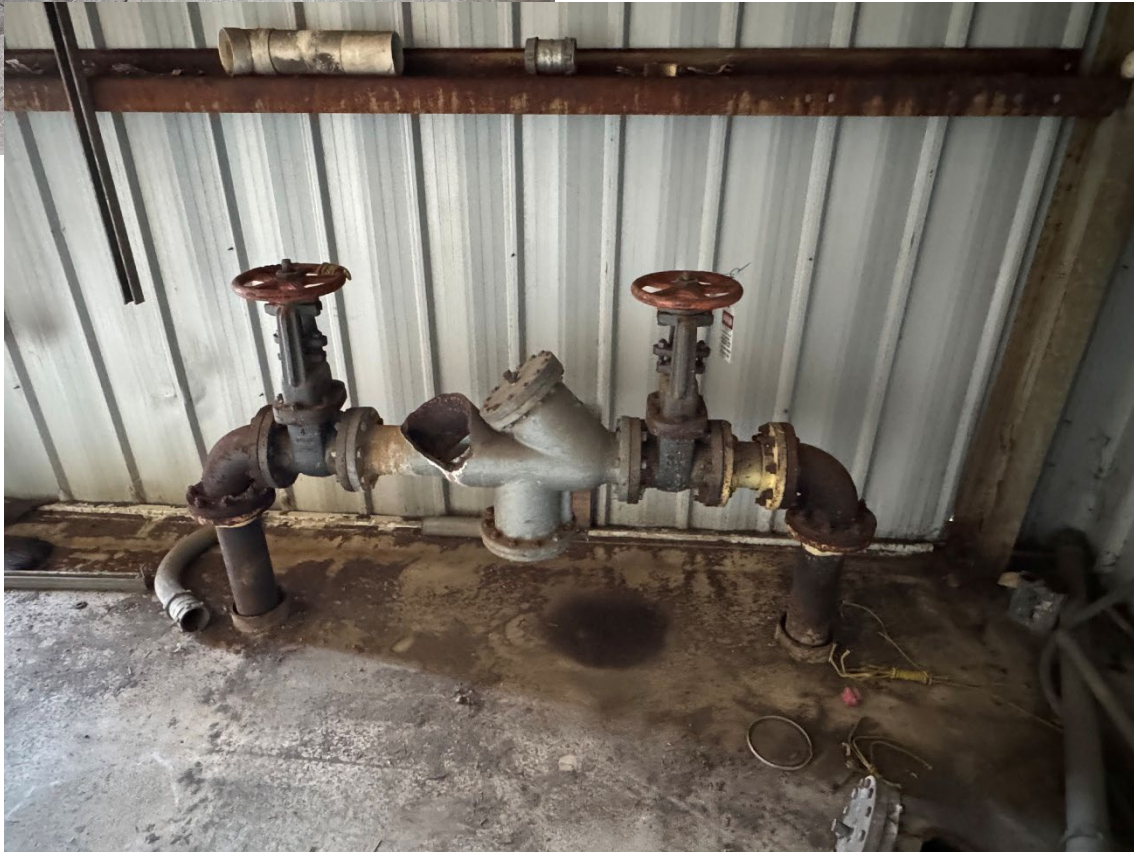
Photo 6 – Pipe riser inside Shed, with AACM gaskets in pipe flanges, and AACM packing inside screw valves. Demolition is planned to slab on grade, which means that this riser would be cut off at concrete. A certified asbestos contractor could cut the riser in-tact, wrap in two layers of 6-mil poly, and dispose as ACM. Other removal methods are also possible.
